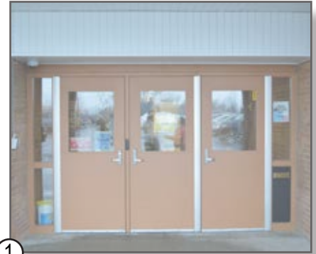
① HOLLOW METAL DOORS & HOLLOW METAL FRAME; STAFF INDICATED CONCERN
