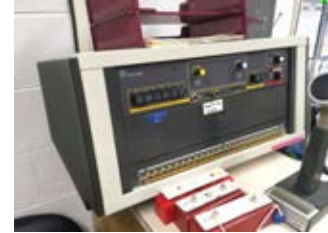
Intercom System Head-End
