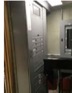
Main Electric Service
