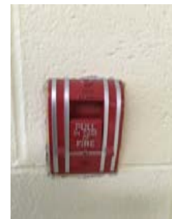
Fire Alarm Pull Station
