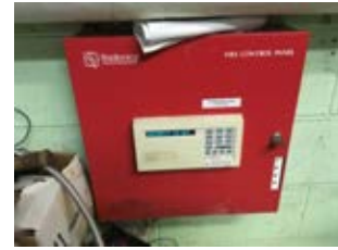
Boiler Monitoring System
