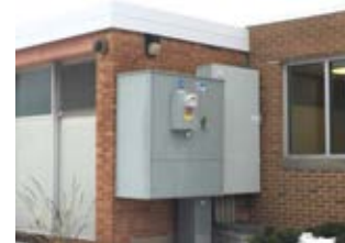
C/T Cabinet & Main Disconnect
